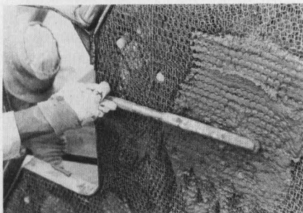
The pencil vibrator is an invaluable tool for ensuring mortar penetration in difficult areas but must be used sparingly.
