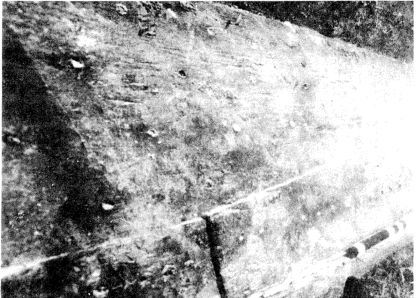
Fig. 13 Photograph of the keel, outer planking and false keel showing the keel joint.
